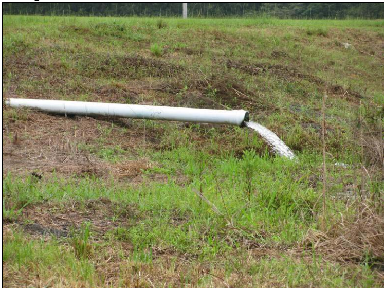
Photo 63: Ash Pond – 8-inch PVC inlet pipe on southeast embankment, looking south. Note: water flowing.
