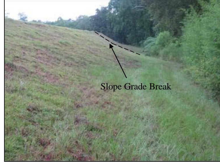
Photo 6: Ash Pond – North embankment exterior slope, change in slope grade from approximately 2.8 H:1V to 2H:1V, looking west.
