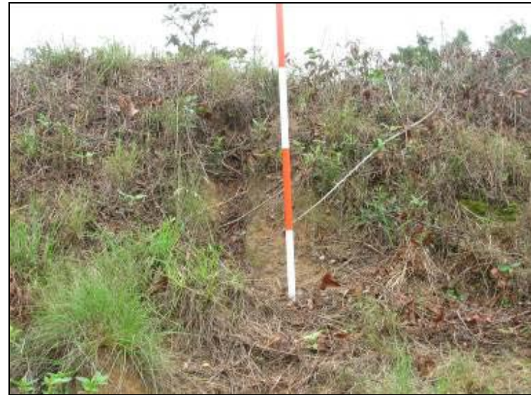
Photo 66: Ash Pond – North Embankment interior slope, erosion rills near outlet structure looking north.
