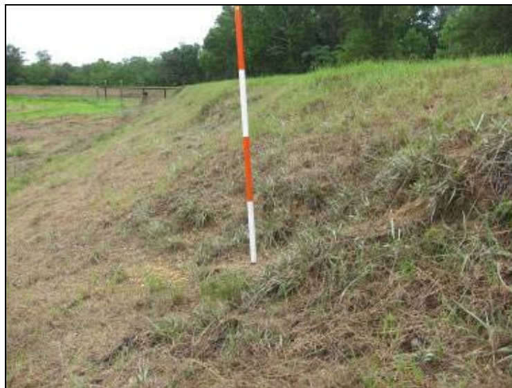
Photo 62: Ash Pond – North embankment interior slope surficial erosion, looking west.
