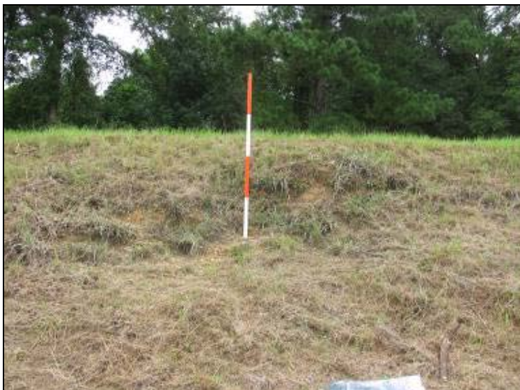
Photo 61: Ash Pond – North embankment interior slope surficial erosion, looking north.
