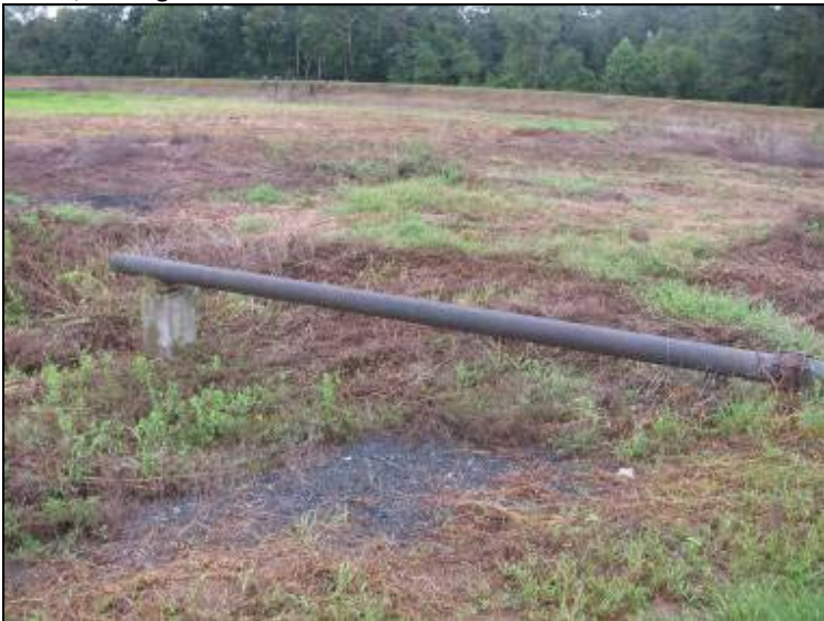
Photo 51: Ash Pond – Southeast embankment interior slope, 7-inch I.D. Ductile iron pipe looking northwest.
