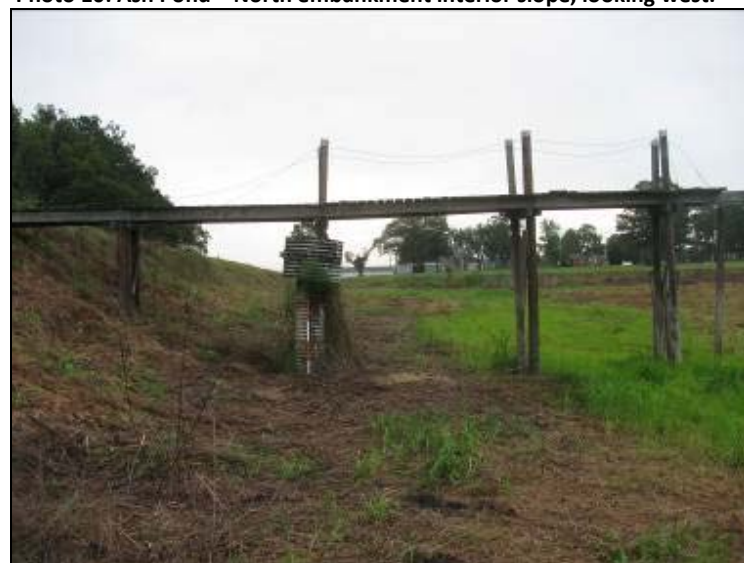
Photo 12: Ash Pond – North embankment interior slope, boardwalk and 18-inch outlet riser pipe looking east.
