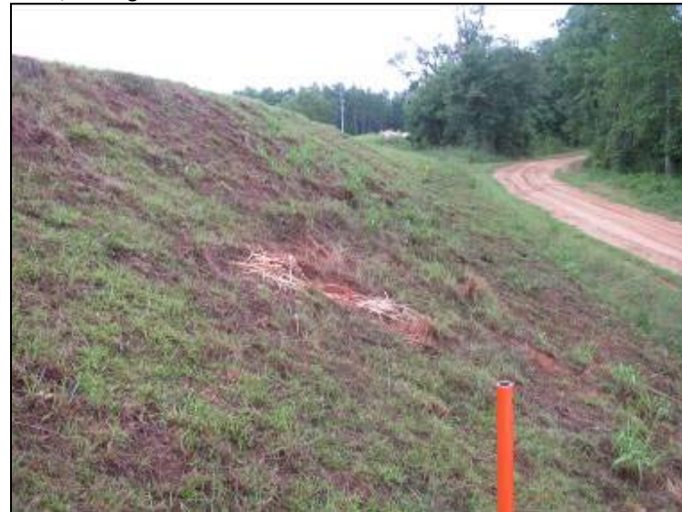
Photo 28: Ash Pond – West embankment exterior slope, looking south. Note: steepness of slope (2H:1V).
