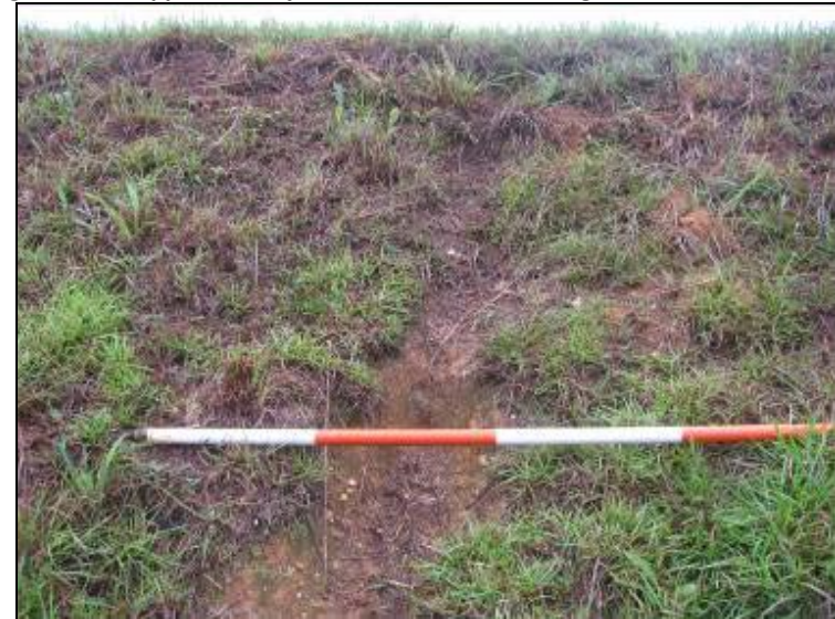
Photo 8: Ash Pond – North embankment exterior slope, erosion rill near crest, looking south.
