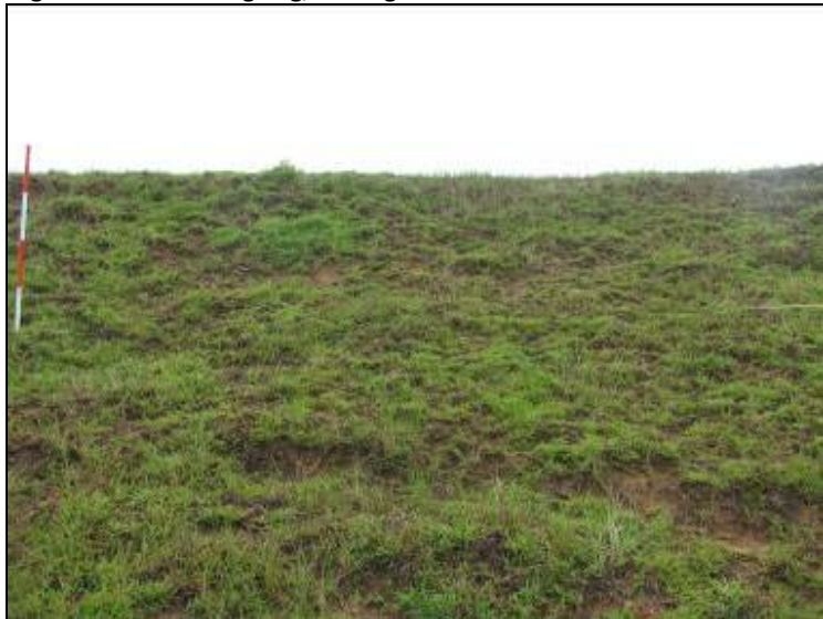
Photo 23: Ash Pond – West embankment exterior slope, apparent 16-foot long semi-circular sloughing, looking east.
