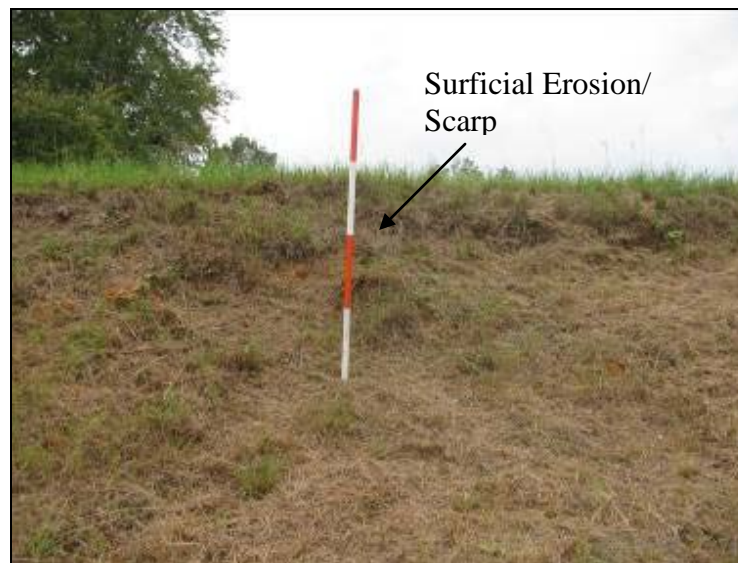
Photo 70: Ash Pond – West embankment interior slope surficial erosion/scarp, looking west.
