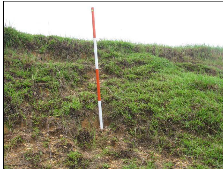
Photo 20: Ash Pond – West embankment exterior slope sloughing, looking southeast.
