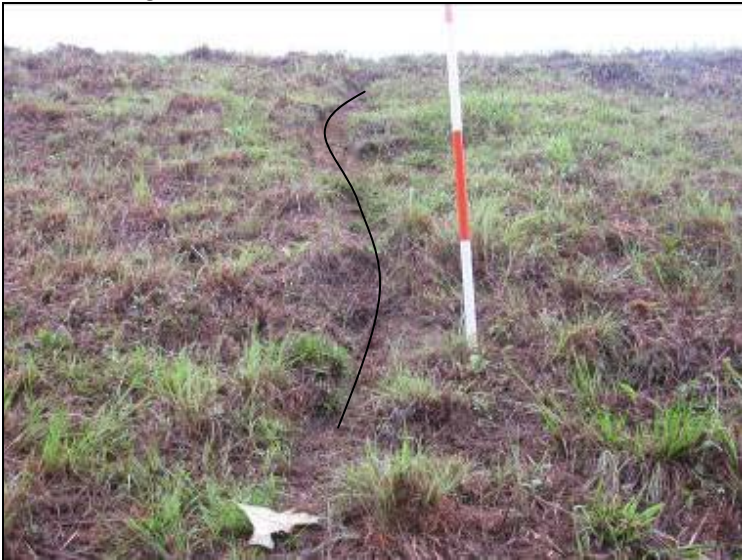
Photo 7: Ash Pond – North embankment exterior slope, surficial erosion rill running from crest to toe of slope looking south.
