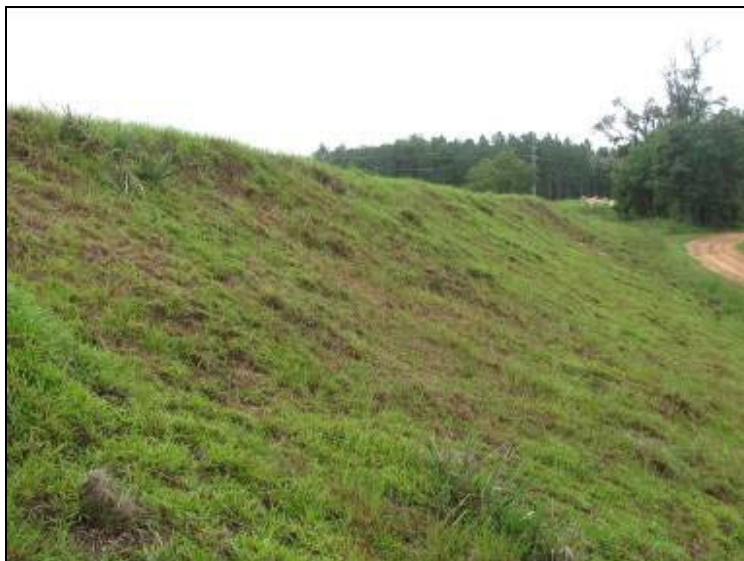
Photo 21: Ash Pond – West embankment exterior slope, apparent 16-foot long semi-circular sloughing, looking southeast.
