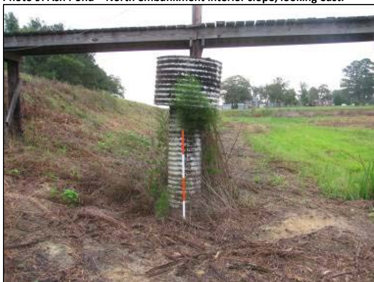
Photo 11: Ash Pond – North embankment interior slope, 18-inch outlet riser pipe, looking east.
