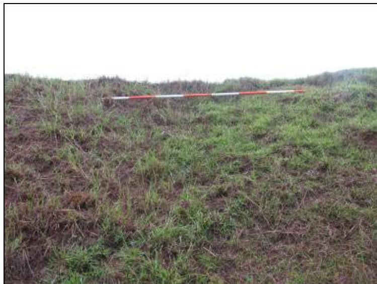
Photo 25: Ash Pond – West embankment exterior slope, sloughing near crest of embankment, looking east.
