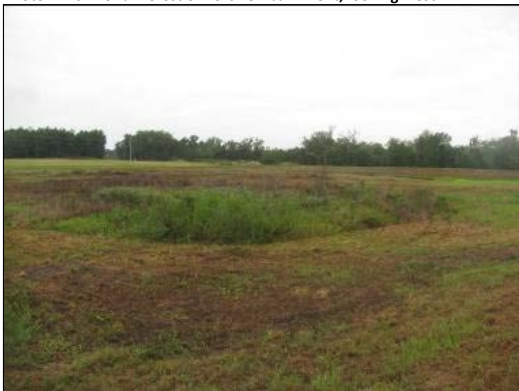
Photo 3: Ash Pond – North embankment interior slope, general view of pond surface area looking southwest.
