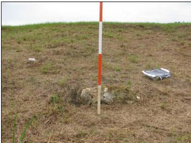
Photo 73: Ash Pond – South embankment interior slope, looking south. Note protruding rock at slope face.
