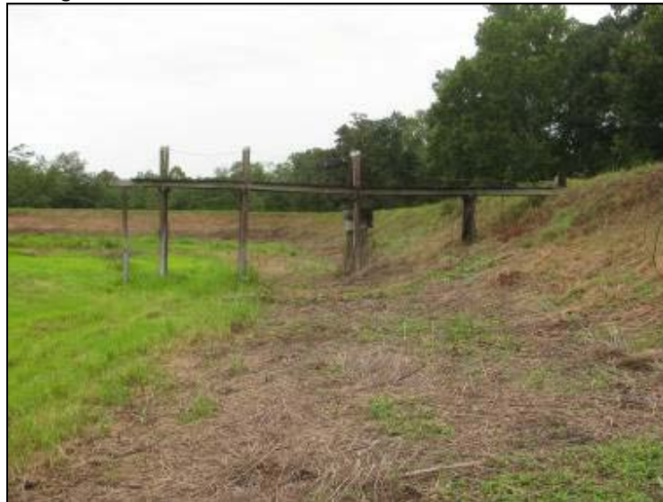
Photo 64: Ash Pond – North embankment interior slope, boardwalk and outlet 18-inch CMP riser pipe looking west.
