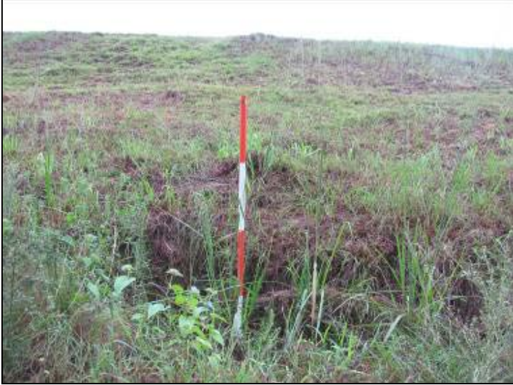
Photo 29: Ash Pond – West embankment exterior slope, swale cut at toe of slope, looking east.
