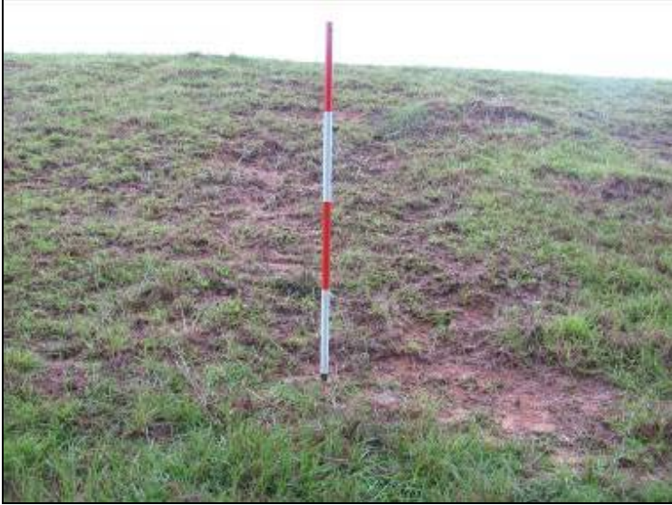
Photo 5: Ash Pond – North embankment exterior slope, minor surficial erosion looking south.
