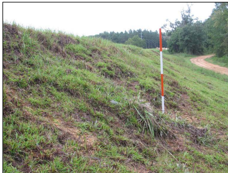
Photo 18: Ash Pond – West embankment exterior slope sloughing, looking South.
