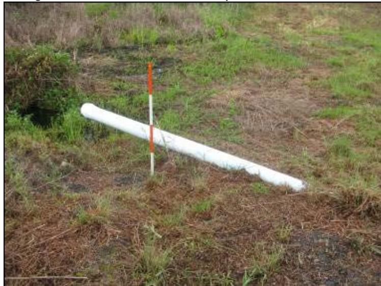
Photo 55: Ash Pond – Southeast embankment interior slope, 8-inch PVC inlet pipe, looking northwest.
