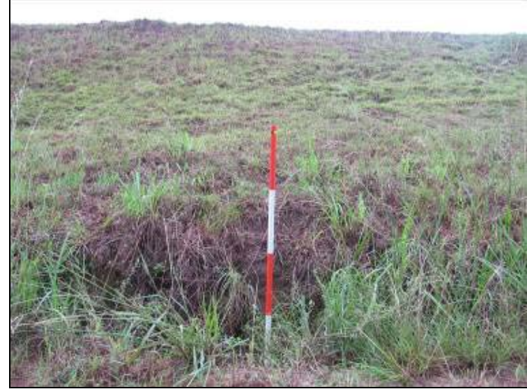
Photo 30: Ash Pond – West embankment exterior slope, swale cut at toe of slope, looking east.
