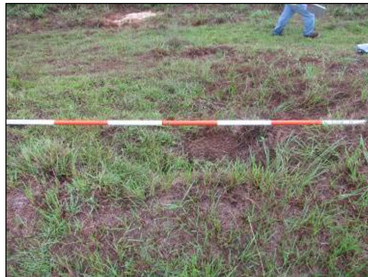
Photo 26: Ash Pond – West embankment exterior slope, sloughing near crest, looking west.
