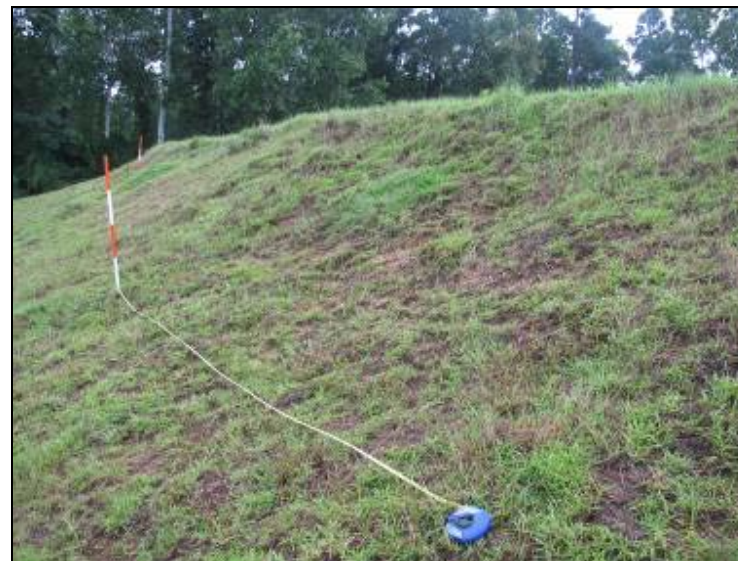
Photo 22: Ash Pond – West embankment exterior slope, apparent 16-foot long semi-circular sloughing, looking north.
