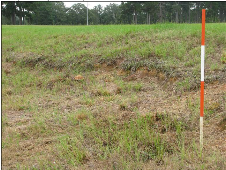
Photo 75: Ash Pond – South embankment interior slope, surficial erosion looking southeast.
