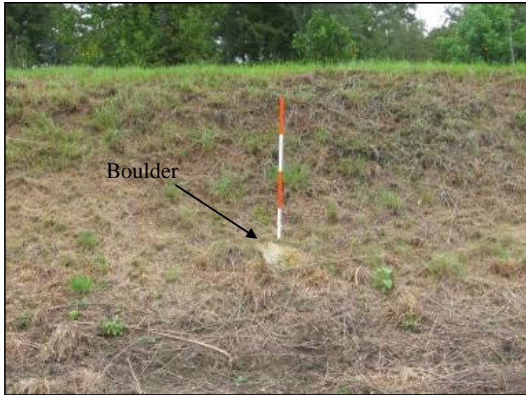
Photo 65: Ash Pond – North embankment interior slope, looking north. Note: boulder (12"-24") and steepness of slope (2H:1V).
