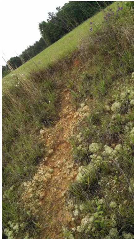
PHOTO 34 ANIMAL PATH ON INTERIOR SLOPE OF S EMBANKMENT
