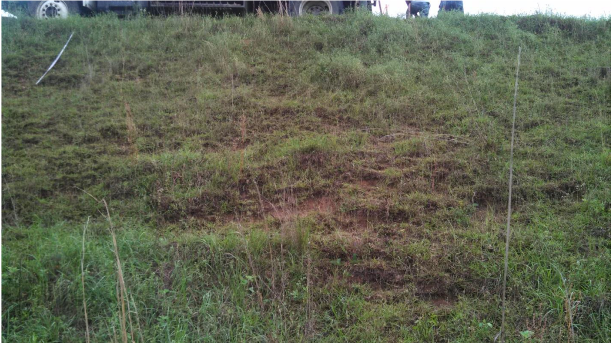
PHOTO 39 W EMBANKMENT BARE/ IRREGULAR EXTERIOR SLOPE (LOOKING E)
