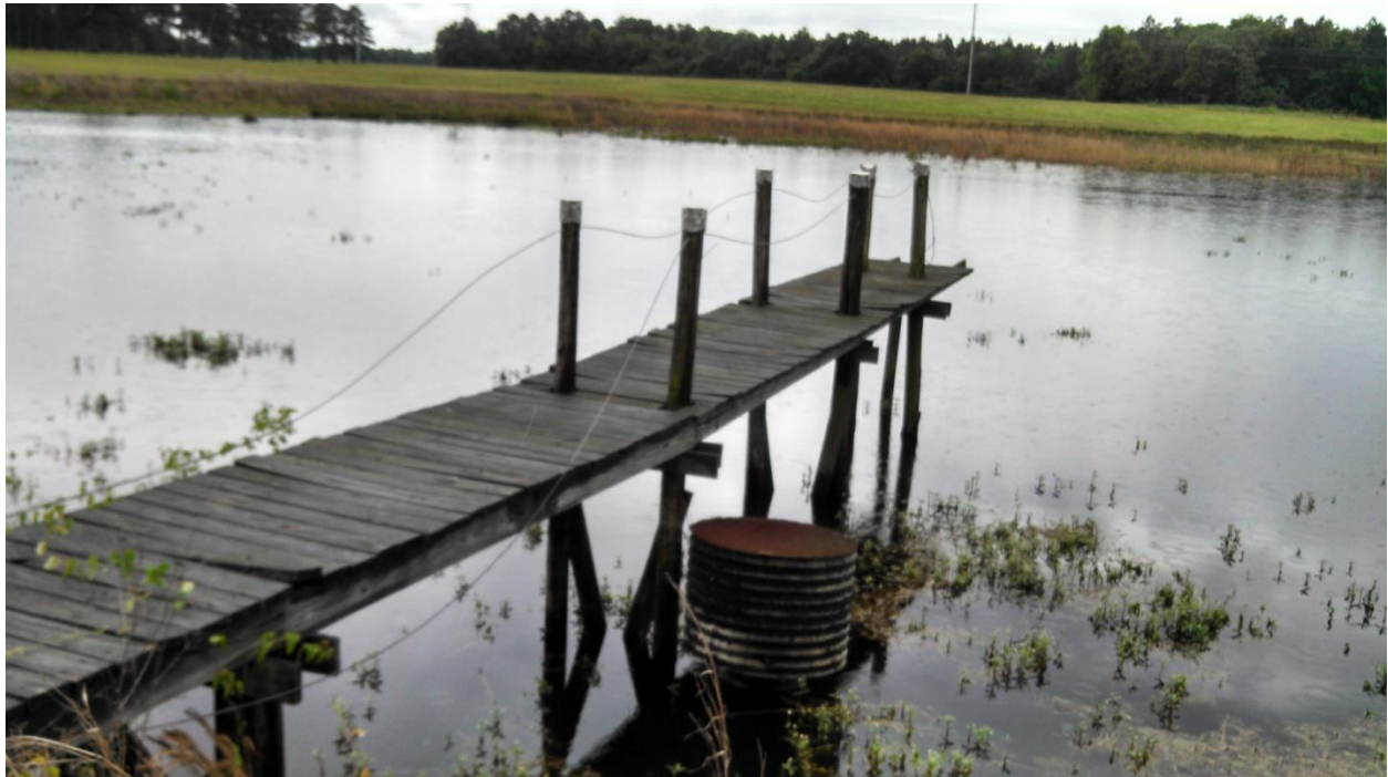
PHOTO 14 BOARDWALK, CMP DROP INLET, AND TRASH SCREEN
