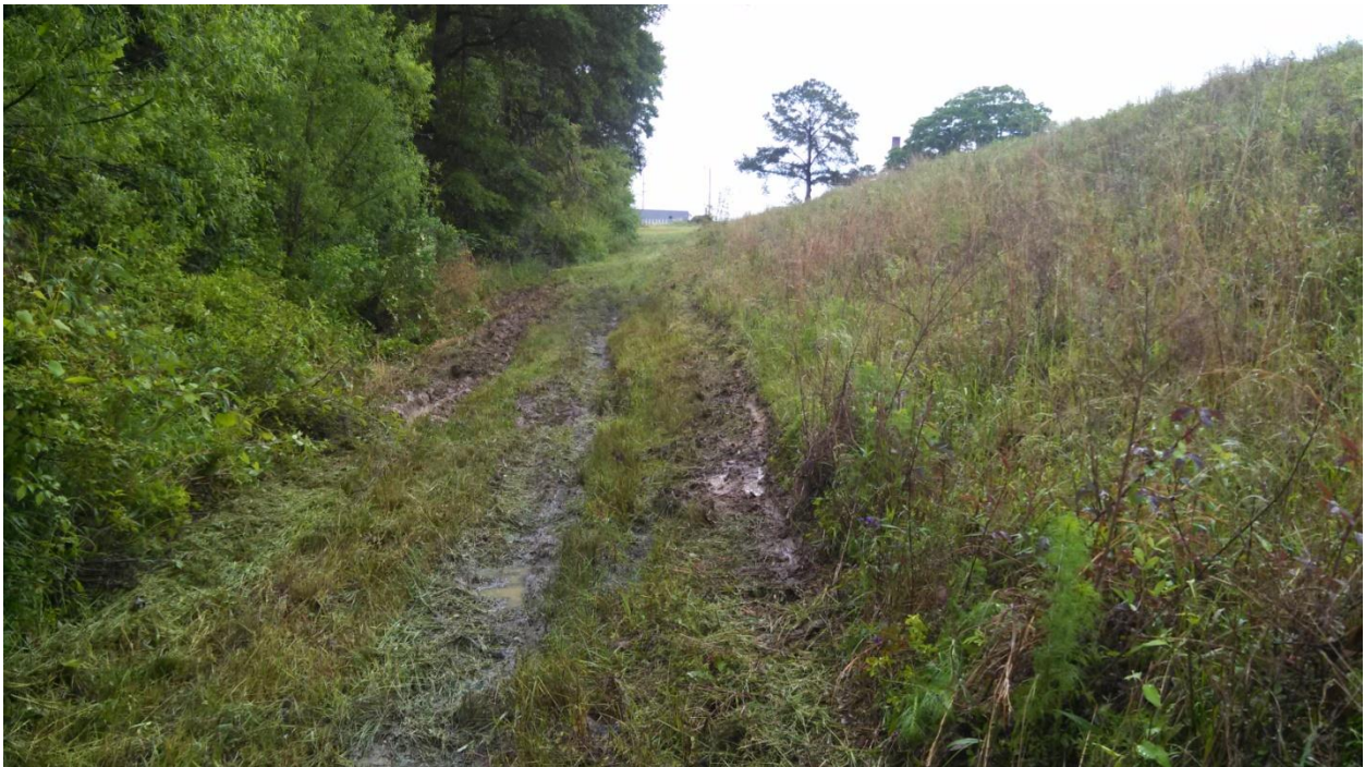
PHOTO 8 EXTERIOR SLOPES, STANDING WATER, AND SOFT AREA AT TOE OF N. EMBANKMENT (LOOKING E)
