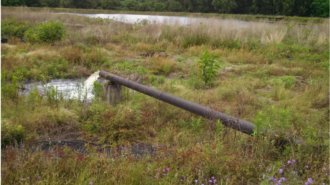
PHOTO 30 7" DUCTILE IRON DISCHARGE PIPE
