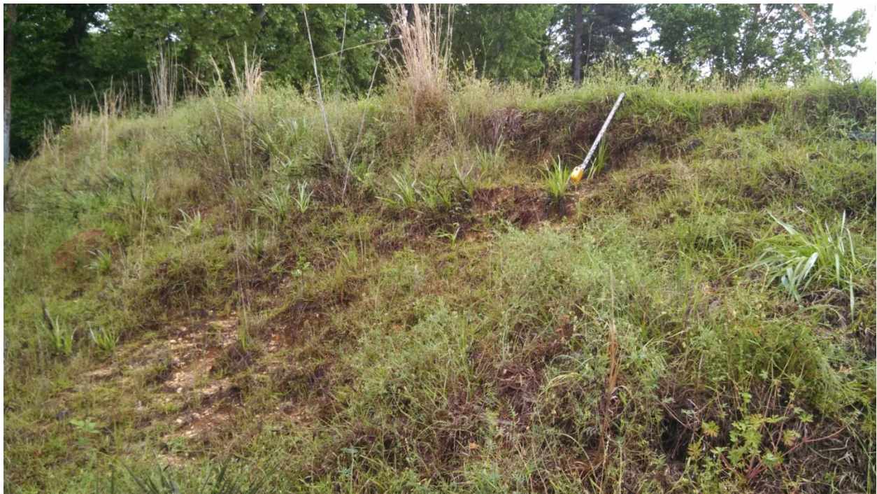
PHOTO 41 IRREGULAR EXTERIOR SLOPES ON W EMBANKMENT (LOOKING NE)
