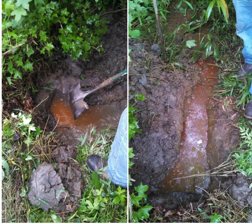
PHOTO 17 RUSTY STORED WATER DRAINING FROM UNPLUGGED DISCHARGE
