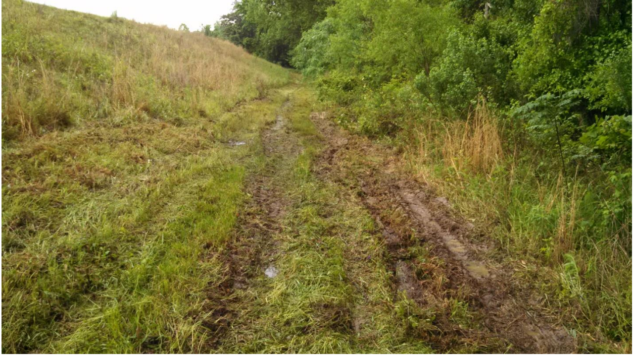
PHOTO 7 EXTERIOR SLOPES, STANDING WATER, AND SOFT AREA AT TOE OF N. EMBANKMENT (LOOKING W)
